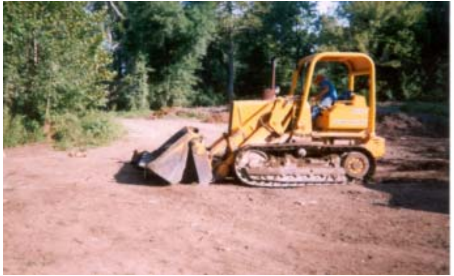
Gravel is best removed from loosely packed bars above the water line. This decreases the potential for increased erosion and still allows a good source of sand and gravel.
